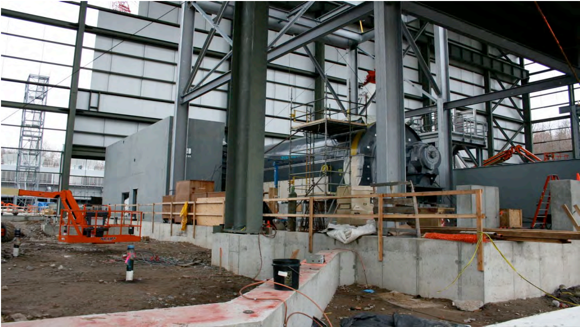
SIEMENS GENERATOR ON FOUNDATION
