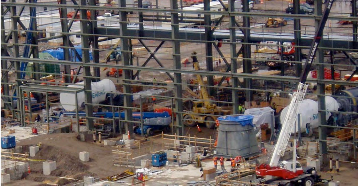
TWO SIEMENS GAS TURBINES INSIDE OF BUILDING
